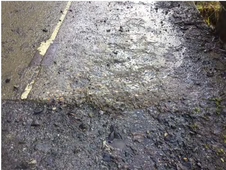
Downstream right bank slab wearing at end
