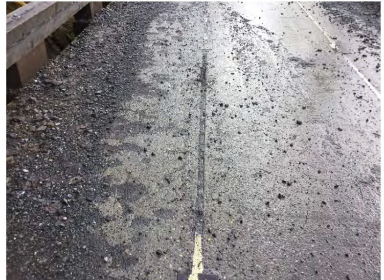
Missing some paraseal
